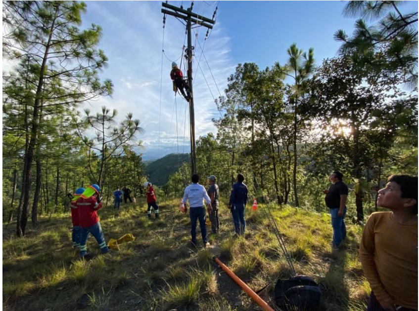
The result of effective conflict management: Electricity was connected again after a process of analysis and dialogue. Photo by: Miguel De Leon
