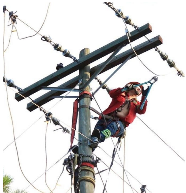
Access to and management of electricity is often a trigger for social conflict: Technician working on electric infrastructure in Santa Cruz del Quiché. Photo by: Miguel De Leon
